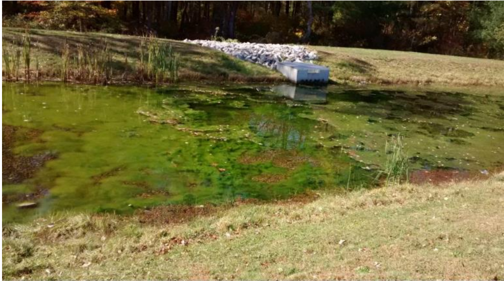
Figure 3a: Stormwater drainage area on Lakeshore Center site with algae bloom (2022)
